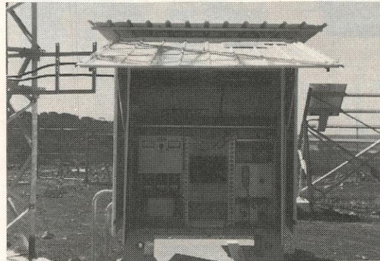
Fig. 19: Equipment Side of Repeater Shelter
