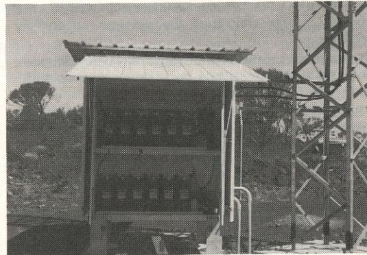
Fig. 20: Battery side of Repeater Shelter
