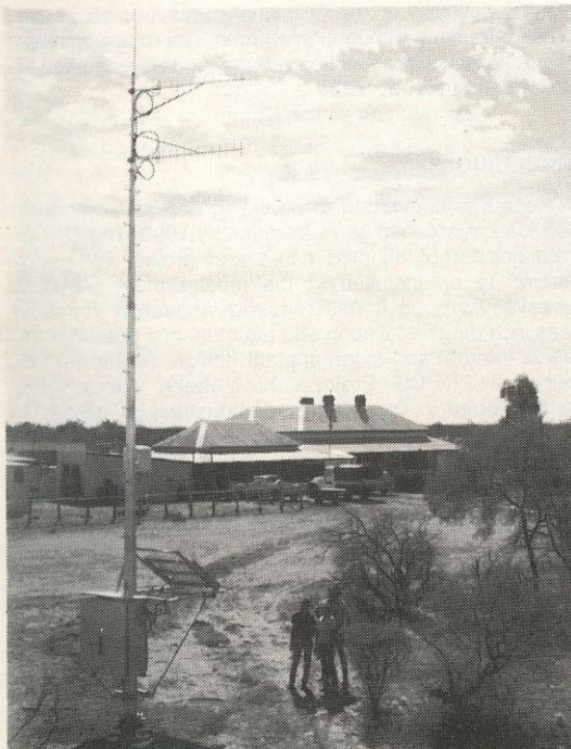
Fig. 18: Customer Equipment at Milly Milly Station
