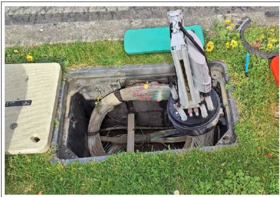
Figure 1. Chorus UFB underground fibre distribution
